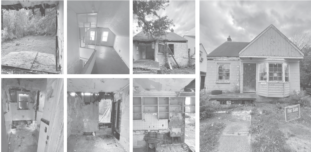
Figures 4.1-4.7: Site photos of DLBA Auction house, located at 15086 Mapleridge, Detroit, MI 48205
