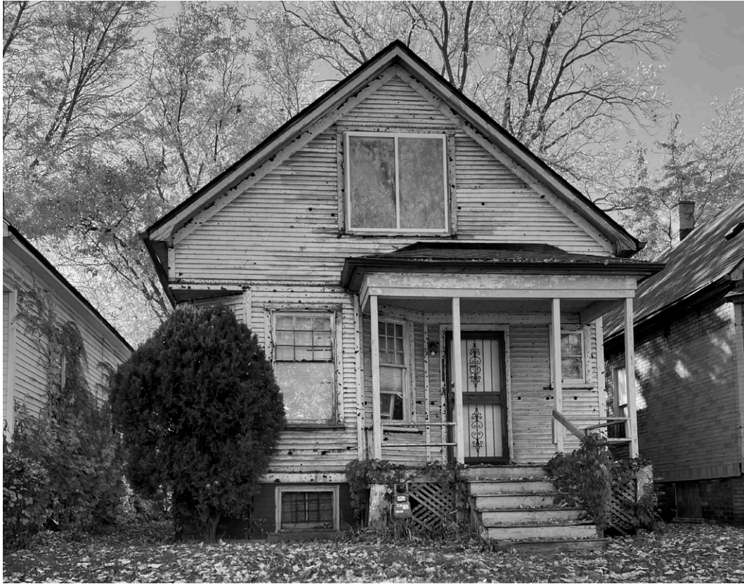
Figure 4.29: Islandview Abandoned house, Single Family
