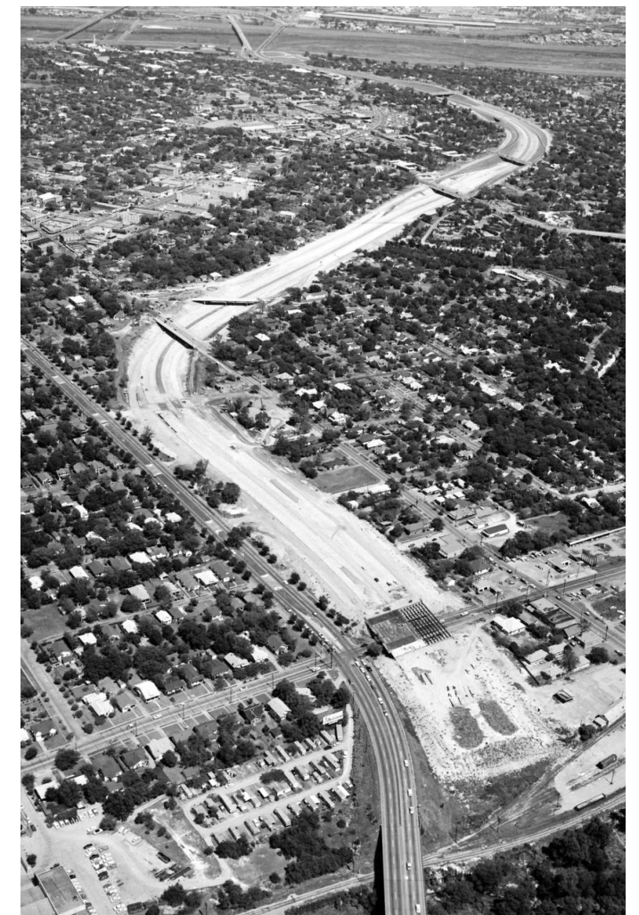
Figure 1.1 Construction of I-35E, 1961. Photo Credit: Tom Dillard / The Dallas Morning News, Retrieved at WordPress.com , 2024, panethos.wordpress.com/wp-content/uploads/2018/04/construction_1961.jpg. Accessed 24 Apr. 2024.
